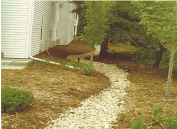
Figure 4.2 An example of an infiltration trench that receives water from roof runoff. Infiltration trenches are most often placed under roadways (source: chesapeakestormwater.net).
