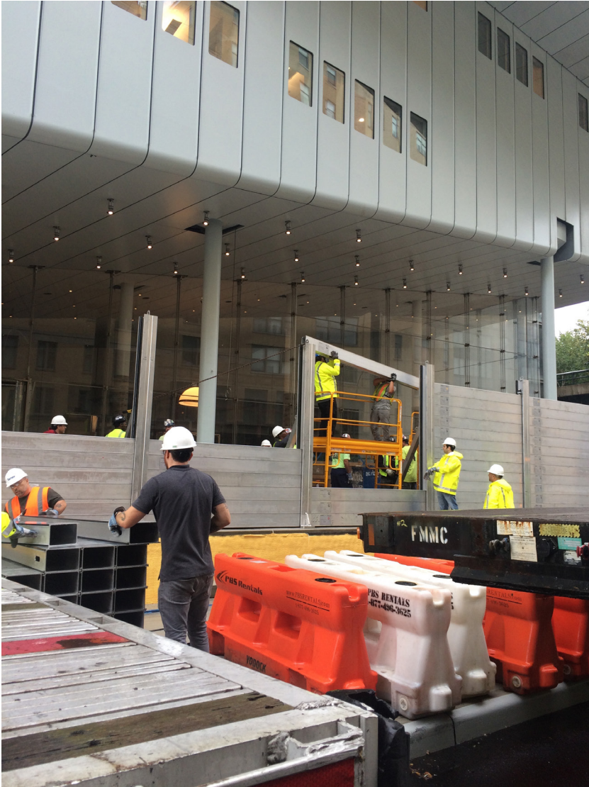
Figure 6.2: Temporary flood barriers for the Whitney Museum of American Art, New York City. The photo shows the structure and method of emplacing the barriers.
