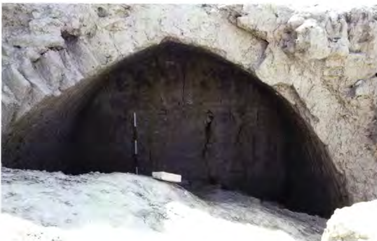
Figure 104 The builders of Merv's traditional houses used a variety of techniques in the same building. In this vaulted room at Suli Köshk [7], the end wall is formed of rammed earth or pakhsa blocks, while the vault is constructed of mud bricks.
