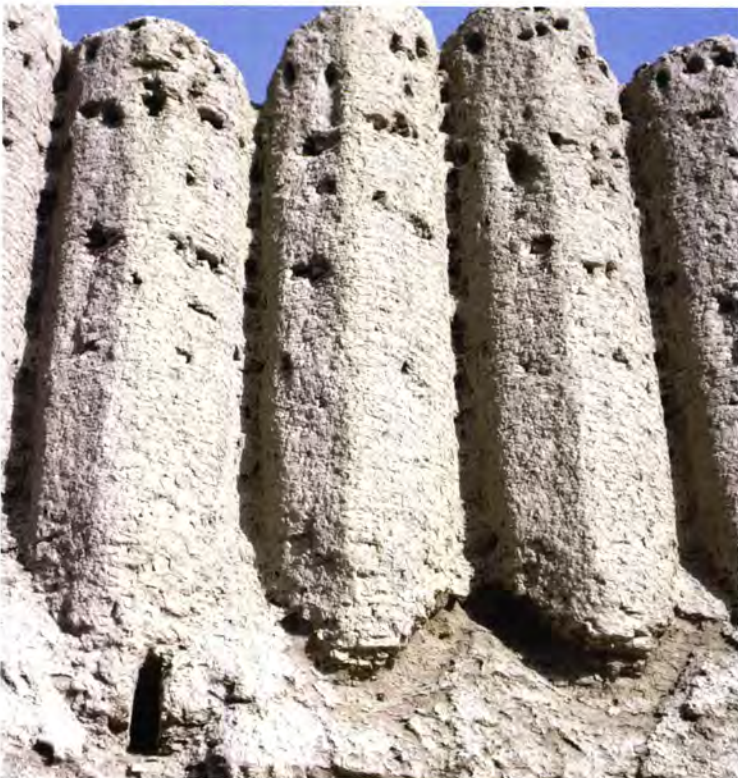
Figure 79 The corrugations of the Greater Kyz Kala [1] are 'tall' corrugations, which continue to the top of the building to form the parapet. While today they are pointed, originally they were probably crenellated. Note the narrow slot of the window lighting the ground floor.
