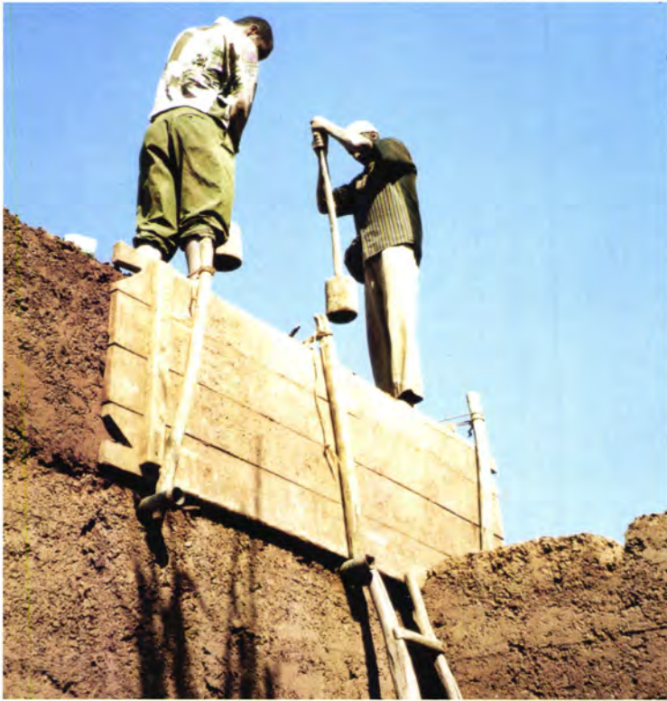
Figure 38 The builders at work on a wall made of blocks of rammed earth. A short section of shuttering is set up, filled with the prepared mixture and rammed to compact the soil, after which the shuttering is moved along to form the next block: three such blocks can be built in a day.
