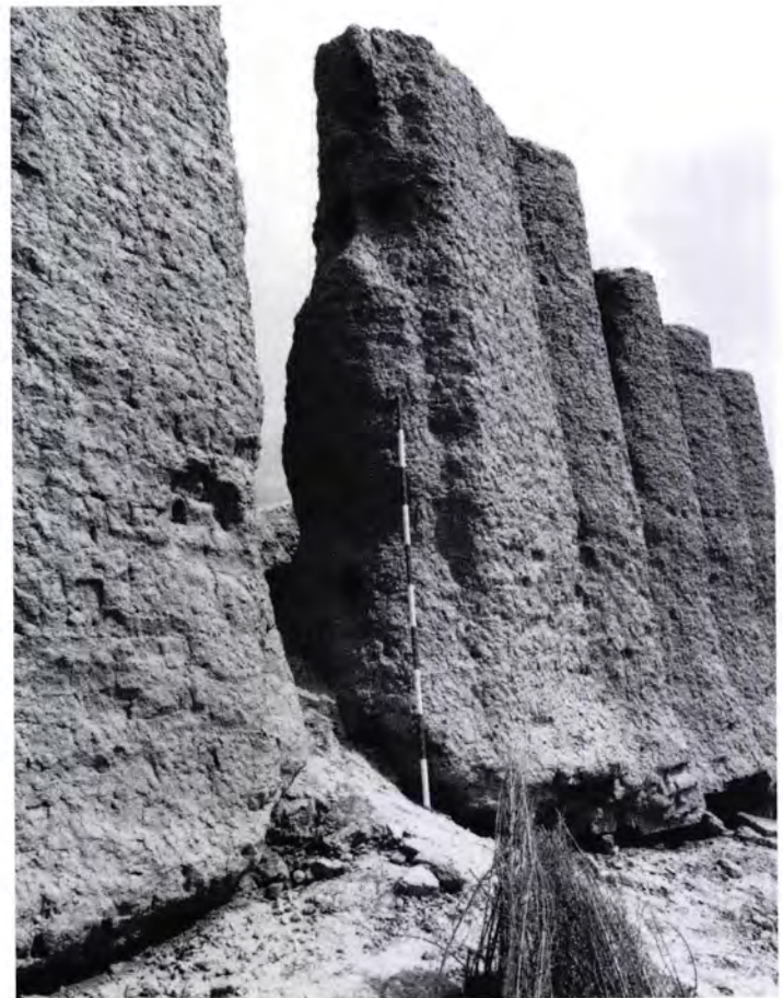
Figure 233 Kyz Kala [13] near Kelte Minar: detail of the centre of the south-west façade with the flattened pilasters and central space, possibly for a window (cf Durnali, Figure 229). Timber beams would have strengthened the gap; note the beam-slots.
