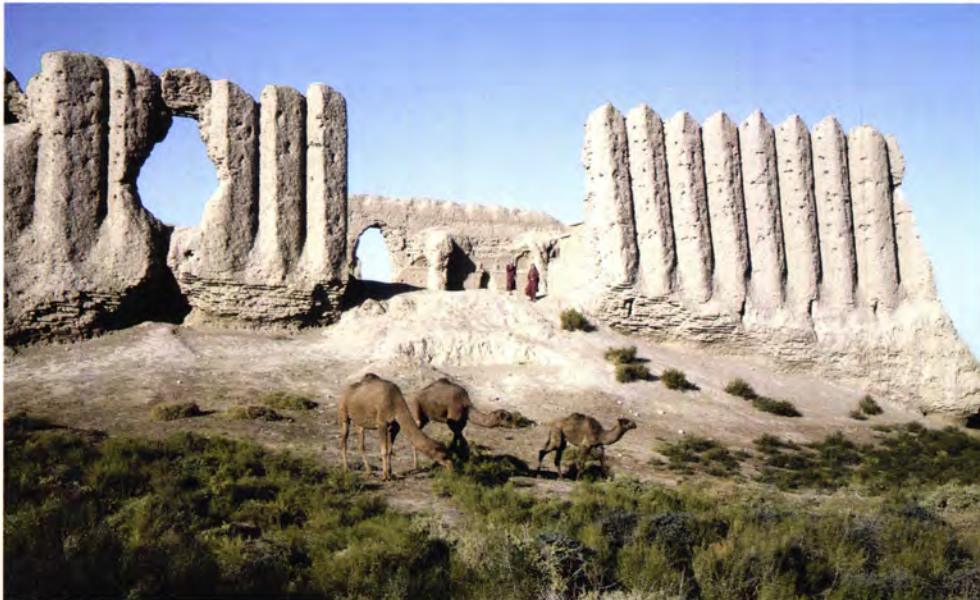
Figure 179 The east façade of the Greater Kyz Kala [1] after the collapse of the central section. Note the additional break on the left and the undercut gullies below. There is no access to the rooms of the lower storey, which were lit by narrow windows. Little survives of the internal arrangements of the upper storey, seen through the central gap. Note the horizontal line on the west wall below the corrugations, which marked the floor of the flat roof.
