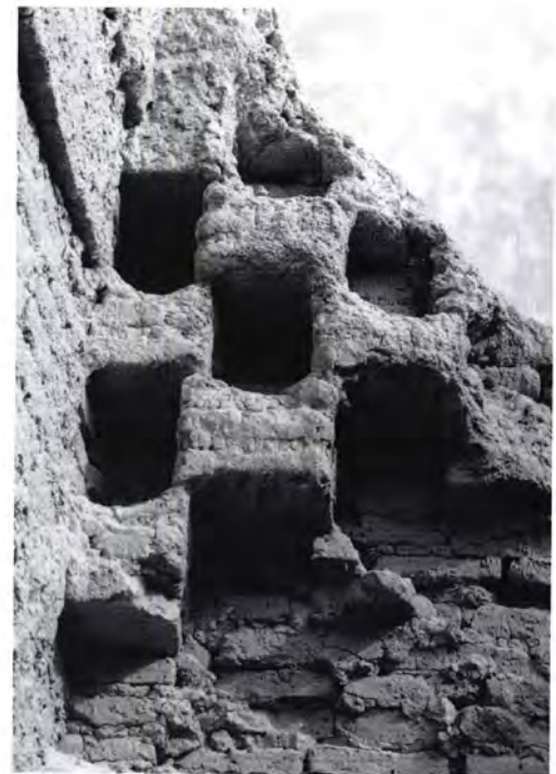
Figure 74 The deep brick niches in the keptar khana [22] in Shahryar Ark, arranged in panels between pilasters carrying the transverse vaults. Many
