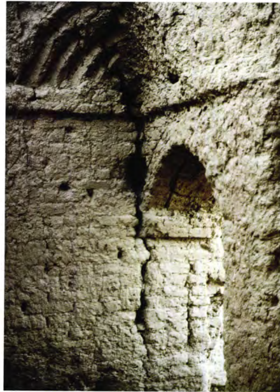
Figure 200 The Lesser Kyz Kala [4]: the north-east corner of Room 8 with the squinch and the arched doorway into the central space or courtyard.
