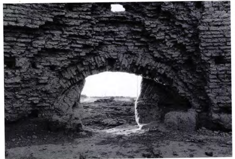
Figure 303 The shallow arch of the doorway of Ice-house 3 [29], on the north west, blocked to reduce its size.
