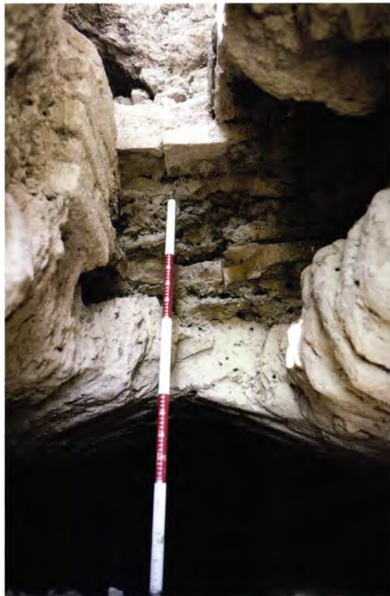
Figure 215 Suli Köshk [7]: a deep crack in the façade has revealed the crown of the vault of a room on the east corner and the floor of an upper-storey room.
