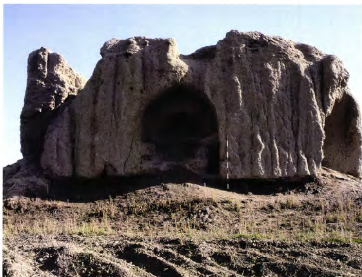
Figure 208 Garam Köshk [6]: the north-west façade with a central iwan. An arched doorway can be seen at the rear of the iwan (Figure 62); collapse on either side has revealed high, barrel-vaulted rooms (Figure 102).
