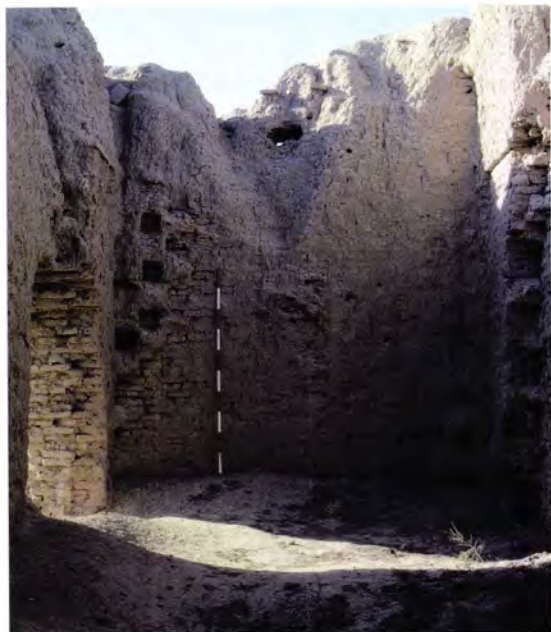
Figure 278 The kepter khana [22] in Shahryar Ark: the south end of the interior. Note the pilaster on the right and the cross vault rising from a course of fired bricks, as well as the remains of panels of niches between the pilasters.
