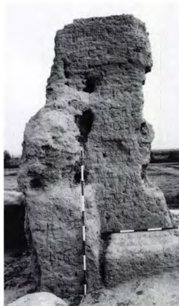
Figure 218 Suli Köshk [7]: the north corner of Room 6. The horizontal ranging rod is resting on the suffa . Above can be seen one of the ventilation slots. Timber beam-slots can be seen in the wall behind the vertical ranging rod.
