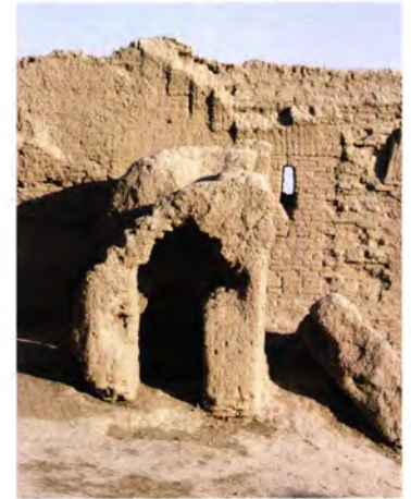
Figure 183 The stairway in the Greater Kyz Kala [1]: the stepped tunnel vault of the flight leading to the lower storey and the springing of a flight leading to the roof. The linking flight has collapsed. Note the small window lighting the stairway.
