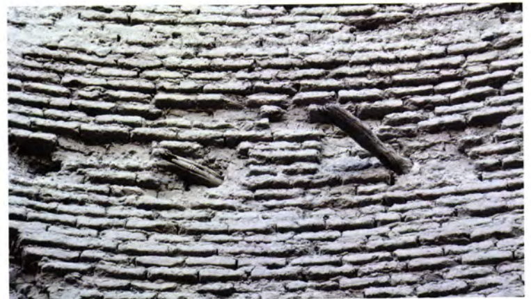
Figure 295 Ice-house 1 [27]: detail of wooden beams projecting from near the top of the interior.
