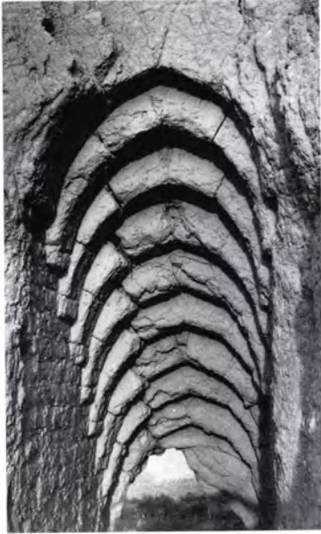
Figure 195 The Lesser Kyz Kala [4]: detail of the stepped tunnel vaults covering the top flight of stairs. The vaults rise from a single brick impost and are formed of curved mud bricks with triangular 'keystones'.
