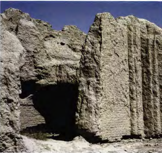
Figure 261 The courtyard walls of the palace in Shahryar Ark [20] were decorated with engaged ribbed pilasters in the corners and along the façades, only a few of which survive. This example is in the north east with Room 3 behind.
