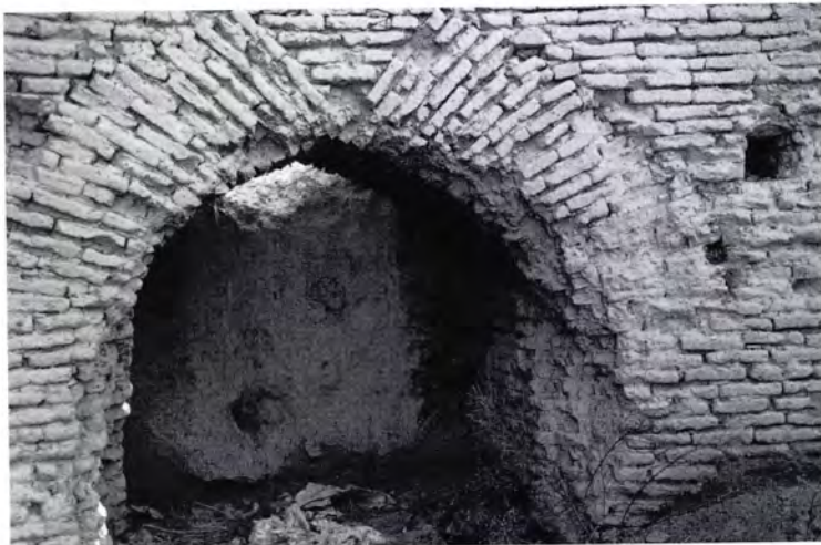
Figure 301 Ice-house 2 [28]: the east niche with its blocking in situ . The arch is constructed of courses of bricks laid radially with a 'keystone' of horizontal bricks.
