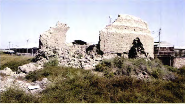
Figure 304 The remains of Ice-house 4 [30] in 1998: a section had collapsed in the preceding winter. The vertical walls and stepped upper section of this ice-house are different from the others.
