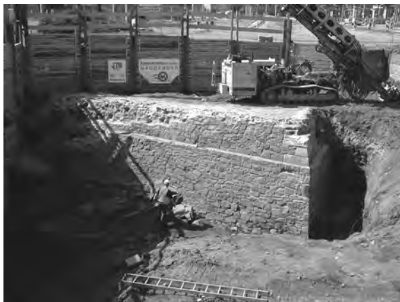
Fig. 17. Magdeburg – Universitätsplatz. The outer point of the Bastion Hessen after its excavation in the course of the construction works for the road tunnel
