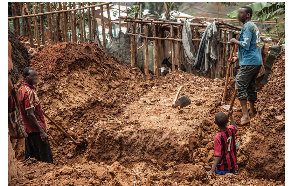
3.1 Two neighbours at Kiziba refugee camp rebuilding an old shelter from scratch on land appropriated outside the camp through negotiations with direct local hosts. Kiziba refugee camp, September 2017. © Amorós Elorduy.
