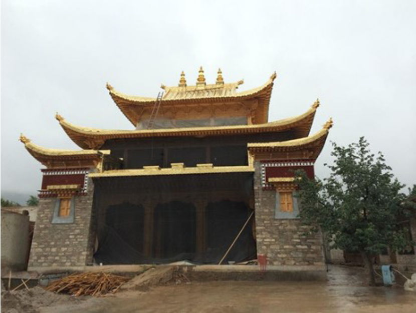
Fig 2.1.b: A new temple under construction in northeast Tibet, 2015. Photo by the author.
