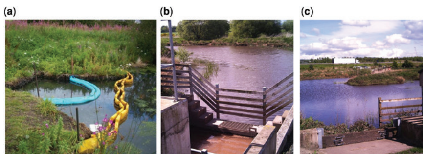
Figure 17.14 Oil spill containment at industrial estate discharge to a retrofit SUDS pond in Livingston, Scotland and (a) contingency design in inlet to treatment pond from swale network and (b) penstock valve at outlet from first pond (c) a timber industries development, Lockerbie, Scotland.
