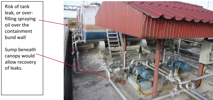
Figure 17.8 Oil storage installation showing inclusion of pump sets within a bunded area, with provision of a canopy to exclude rainfall.
