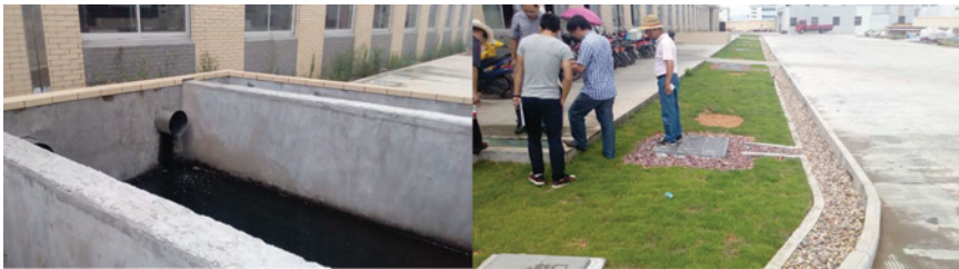
Figure 8.8 Rainwater harvesting system: pre-treatment and storage tank.
