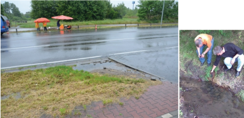
Above: under-drained grass swale under investigation for long term effectiveness at Hoppegarten (photo credit Harald Sommer). Below: Original outlet from Hoppegarten development: still the only discharge point to small receiving watercourse.
