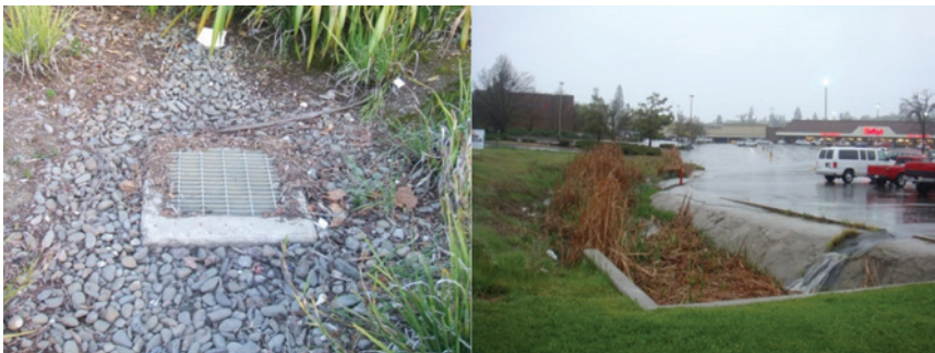
Figure 12.2 Bad management: overflow pipe in bioretention ( above left ) and small constructed wetland ( above right ) blocked with litters (San Francisco/California).
