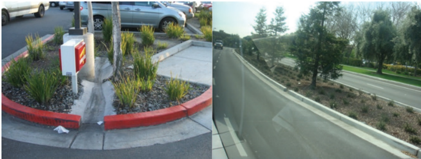
Figure 12.1 Bad design: flow channels were not properly designed so runoff cannot be diverted into the facilities for infiltration (San Francisco/California).
