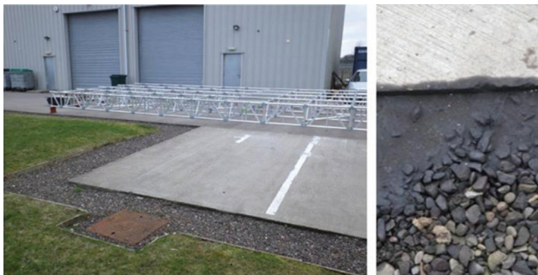
Figure 17.17 Surface drainage using gravel trenches allows for easy detection of poor practice disposal and leaks. Also provides a first stage of degradation for lesser levels of contamination by microbes on the gravel.
