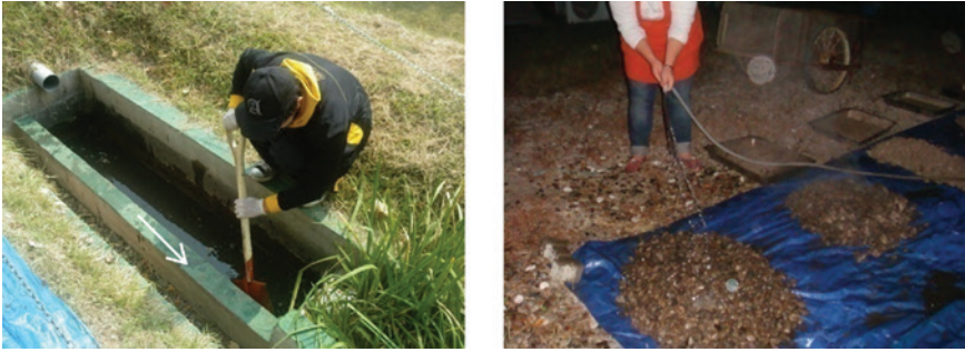
Figure 12.10 Filter media were collected and washed as part of the non-routine maintenance.
