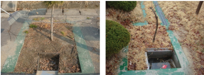
Figure 12.3 Part of the routine maintenance performed in the tree box filter was the inspection of possible accumulation of large debris and litters ( above left ) and checking of standing water and possible clogging ( above right ).
