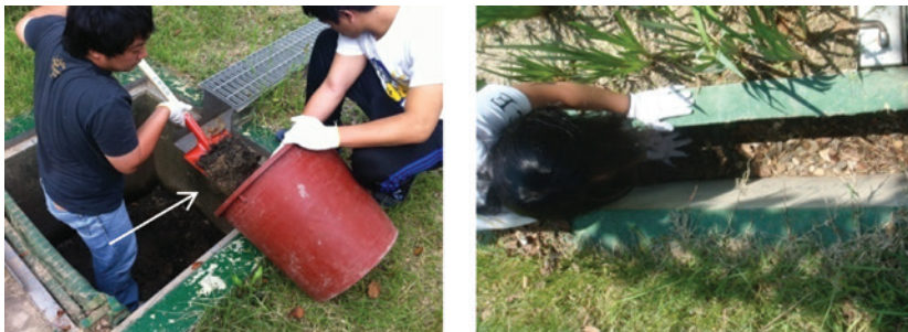
Figure 12.8 Sediments accumulated in the pre-treatment tank of the infiltration trench ( above left ) and overflow area of the hybrid constructed wetland ( above right ) were removed as part of the non-routine maintenance.
