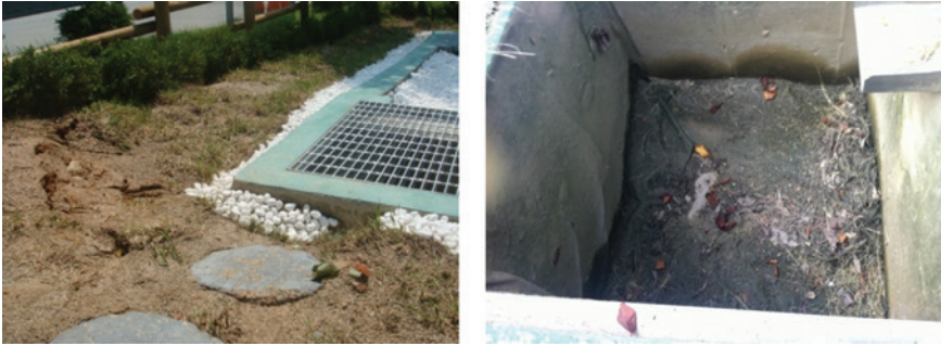
Figure 12.4 Soil settlement ( above left ) and geotextile clogging ( above right ) were also inspected as part of routine maintenance for the infiltration trench.
