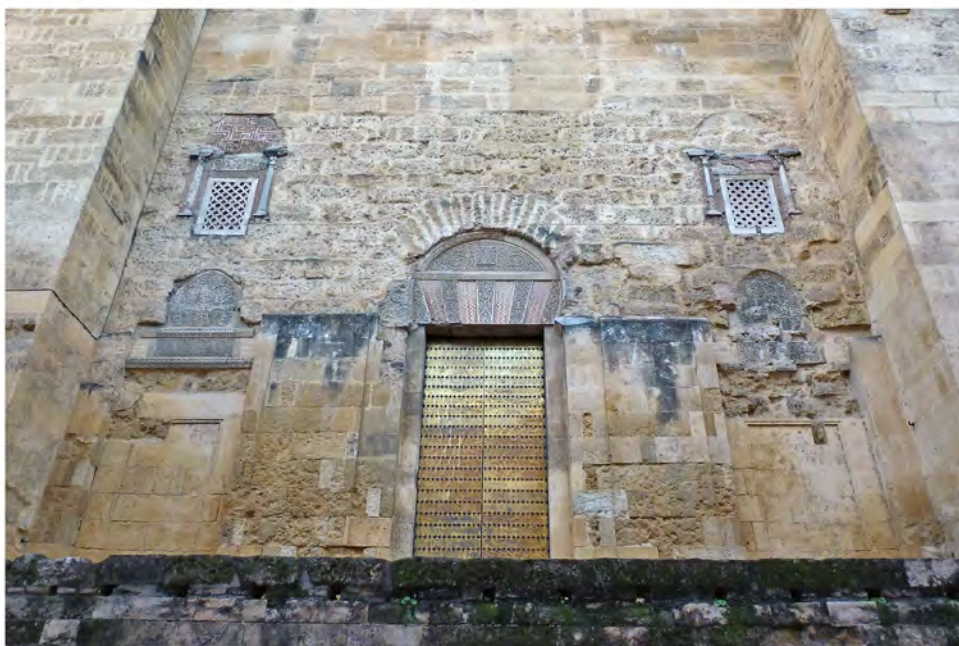
FIGURE 68 Āmirid eastern façade: Gate 1: view and detail of inscription in archivolt © MARIAM ROSSER-OWEN
