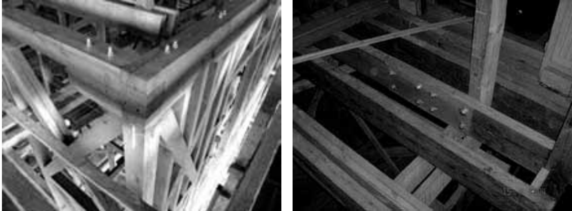
Figure 12. Reinforcing the joints of the timber buildings using mechanical fasteners (Can Binan's archives).
