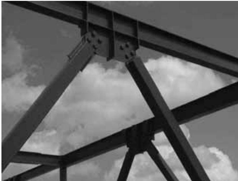
Figure 2. Detail of the HFIR's structure; posts and beams are connected by bolts and nuts.
