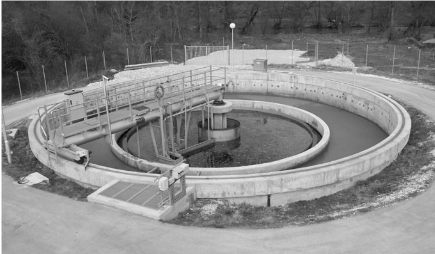
Figure 2. Aeration and sedimentation tanks at Makedonski Brod WWTP.
