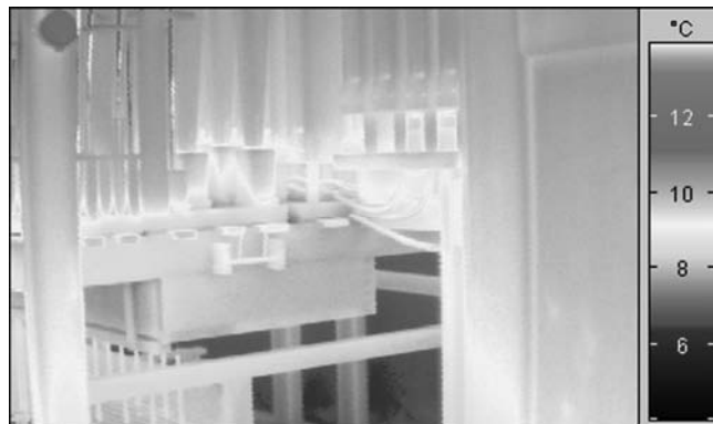
fig. 7: Infrared thermograph of the area from fig. 6
