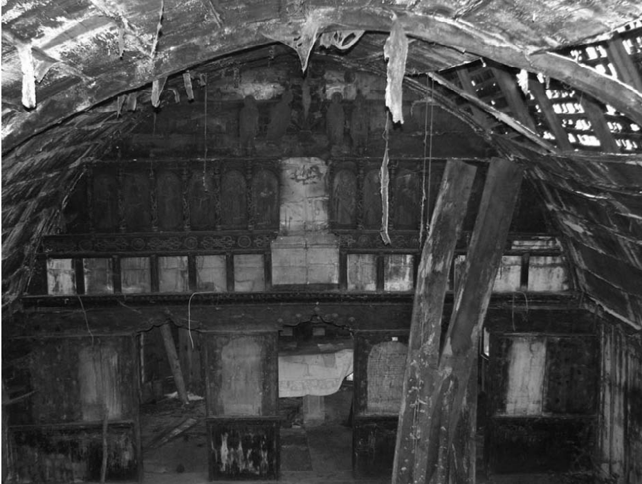
Fig. 6 Vault in collapse
