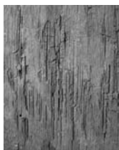
Fig. 5 – Wet rot with cuboidal cracking.
