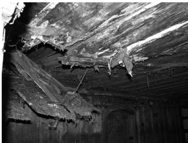
Fig. 4 Vault decayed by the Coniophora puteana and other fungi
