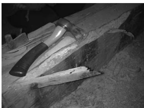
Fig. 7. RP, attack by Old house borer
