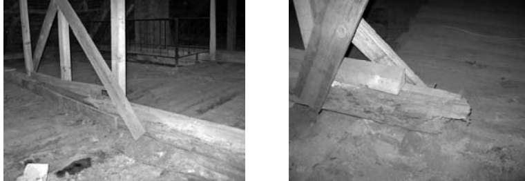
Fig. 7. Wood in the lower chord of the main frame and in the longitudinal tie beam completely destroyed.
