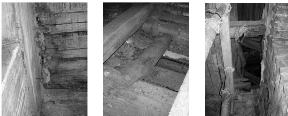
Fig. 10. Floors in the attics: brown rot on the supports, complete destruction of beams.
