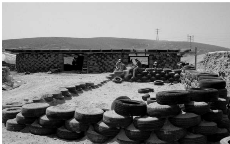
Costruzione della scuola a Khan al Abmar, Territorio Occupato Palestinese, 2009. Tecnica Earthship. / Construction of the School in Khan al Abmar, Occupied Palestinian Territory, 2009. Earthship Technique.
