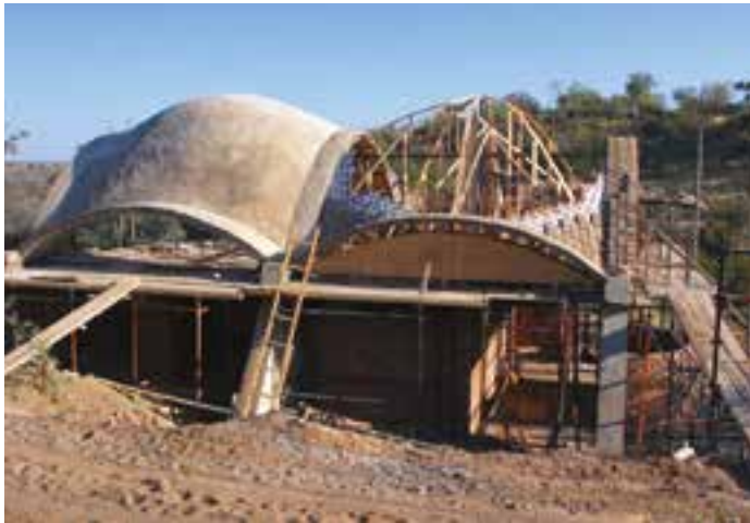
Fig. 11 Mapungubwe Interpretation Centre while being erected with local craft and materials. Limpopo, South Africa. (photo: J. Bellamy)
