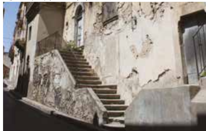
Fig. 10 External staircases lower the centre of gravity of the building and reinforce its base Ragusa, Sicily, Italy (photo: L. Dipasquale).
