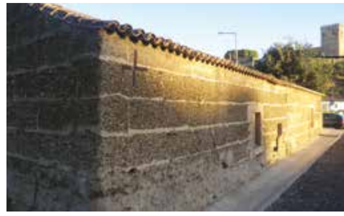
Fig. 5 Anchor plates in a rammed earth building, Mertola, Portugal (photo: M. Correia).
