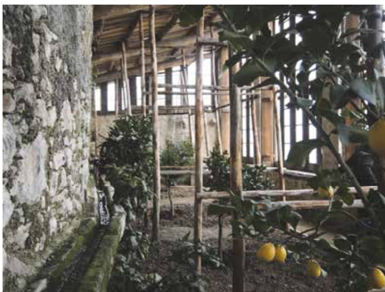
Figure 2 - Inside a recently restored limonaia in Gargnano in Winter months: the limonaia is closed and covered. The irrigation system and many features of traditional citrus fruit growing may be recognized.
