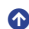
The current wall condition of the tower of "Monte Lucio" – (Pictures, 2018 © Davide Prati & Simone Garagnani).
