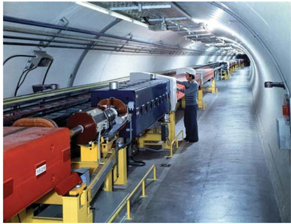
Fig. 3.17 Inside the tunnel housing the Super Proton Synchrotron (SPS) in CERN. The blue blocks are quadrupoles and the red blocks are bending magnets. All magnets are conventional ferromagnets. Photograph copyright CERN
