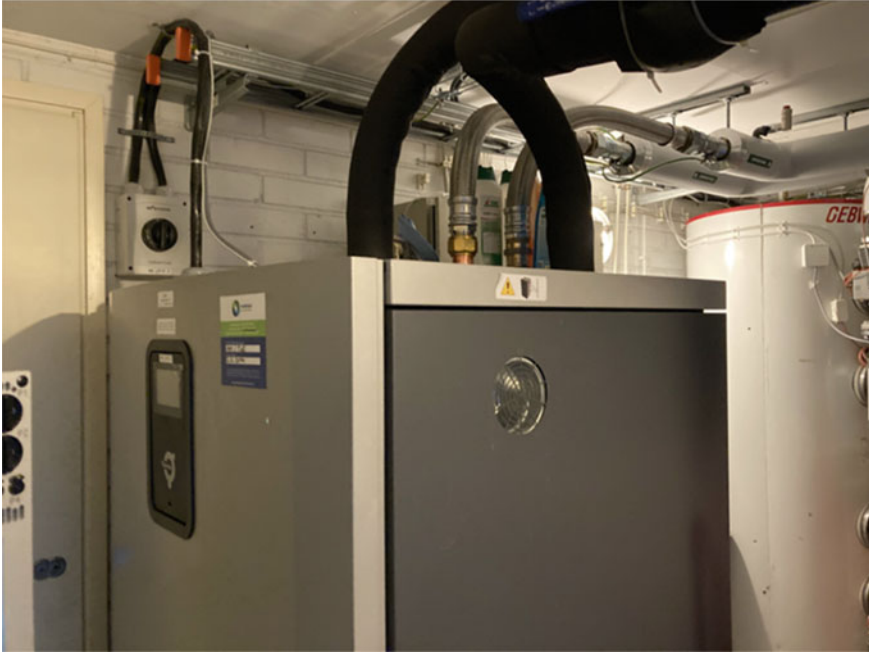
Fig. 7.5 Finnish demo site boiler room with the new heat exchanger
