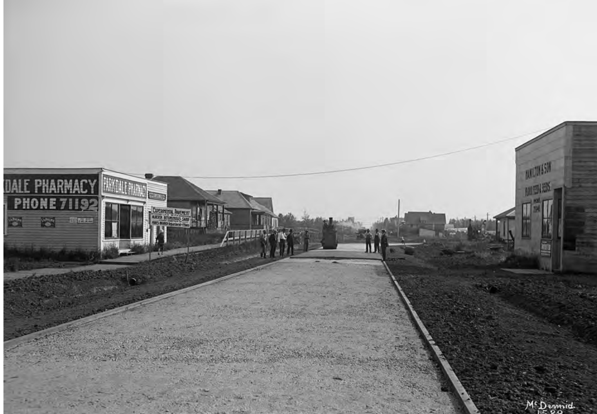
Experimental asphalt paving in Edmonton, Alberta, in 1915 using tar sands from Fort McMurray. McDermid Studio, Glenbow Archives, NC-6-1522.
