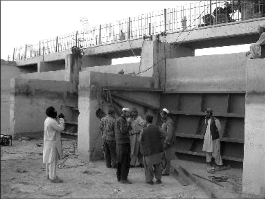
Figure 3: The repair of the Dahla Dam and the Arghandab Irrigation Rehabilitation Project was a key Canadian priority, which aimed to create jobs, transfer knowledge, build capacities, and ensure sustainability in water allocation and agricultural development for Kandaharis. (Credit: CIDA/Lisa Vandehei)
