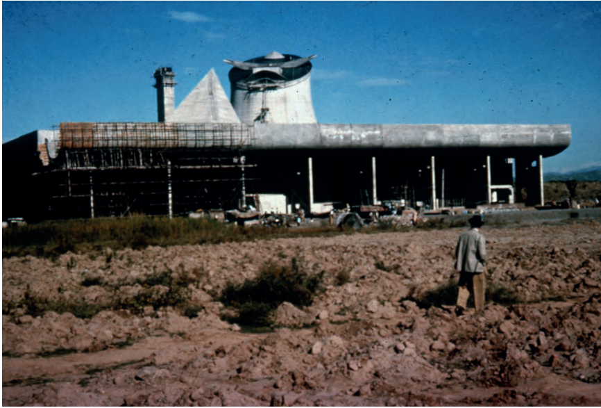
Fig. 270: Le Corbusier on the Construction Site of the Palace of Assembly, Chandigarh, India, 1955-63.
