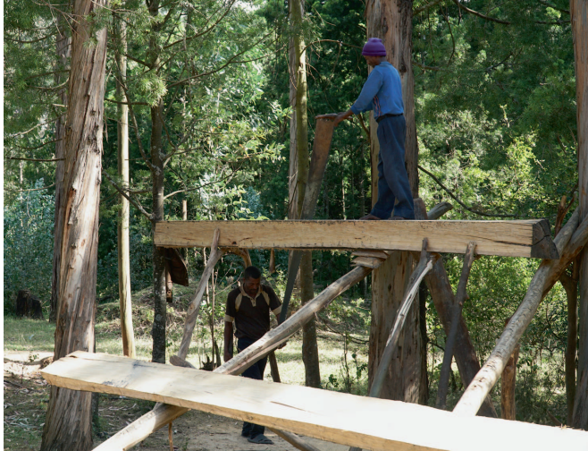
Many things are still done by hand in Ethiopia, e. g. sawing eucalyptus logs into boards
