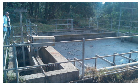
Defective sewage treatment plant in September 2013
