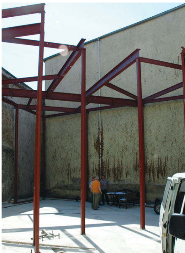
Fig. 15: Braunschweig Synagogue during the erection in a courtyard (Photograph: Ulrich Knufinke, Bet Tfila – Research Unit for Jewish Architecture, Braunschweig, 2006).
