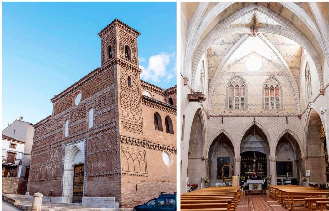
Fig. 01. To the left main portal of the Church with brick walls placed with rope and stick; to the right interior of the main nave and view of the chancel. Grupo de Investigación en Arquitectura (GIA) T37_17R.
