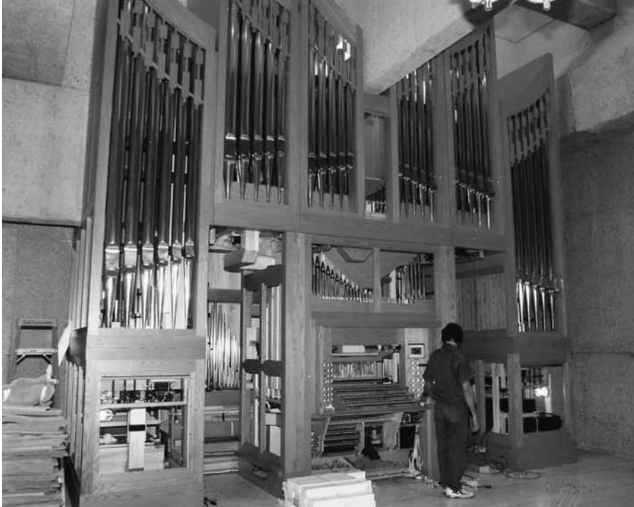
Construction underway on the Carthy Organ at Mount Royal College, 1996. Photographer Mike Ridewood; Mount Royal University Archives E96-22.
