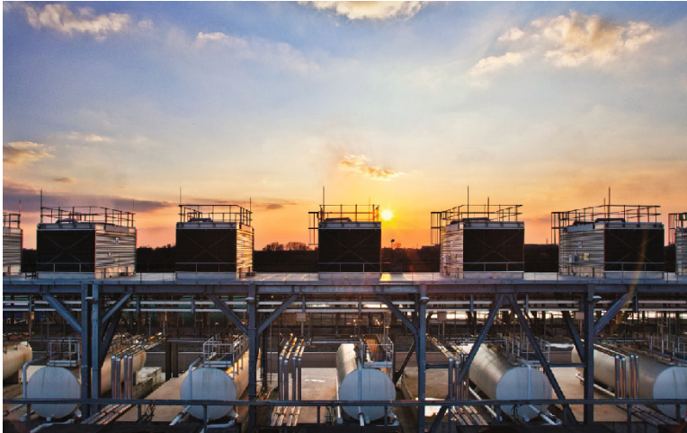
Figure 1.5: Cooling towers and water storage tanks, Lenoir, North Carolina, U.S.
