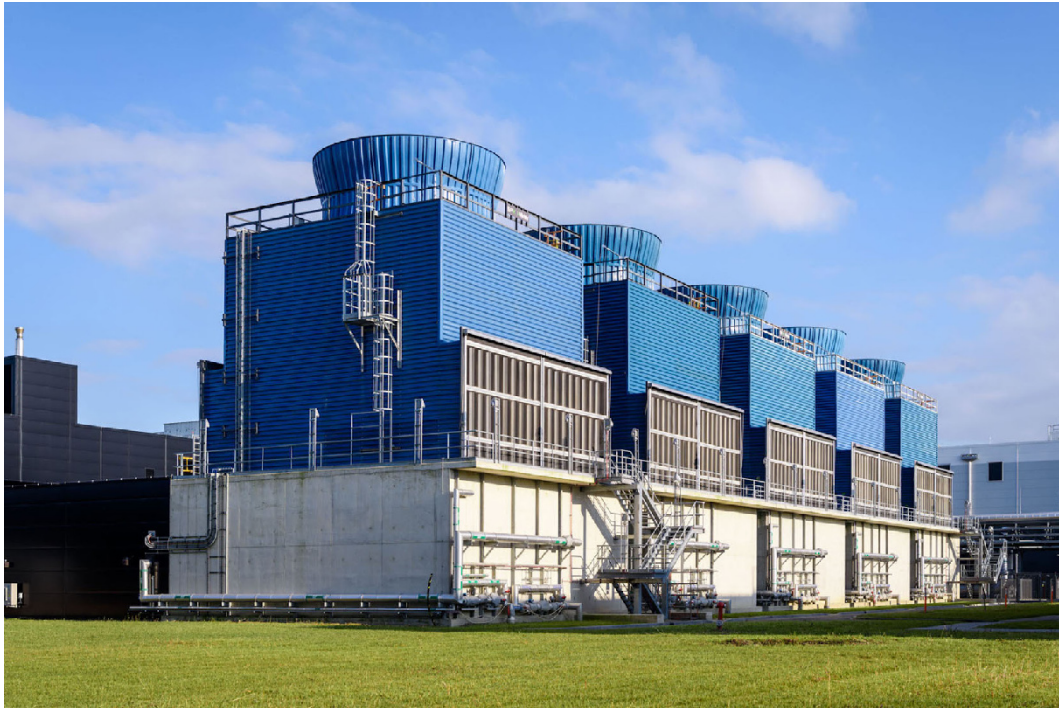
Figure 4.12: Data center cooling towers.
