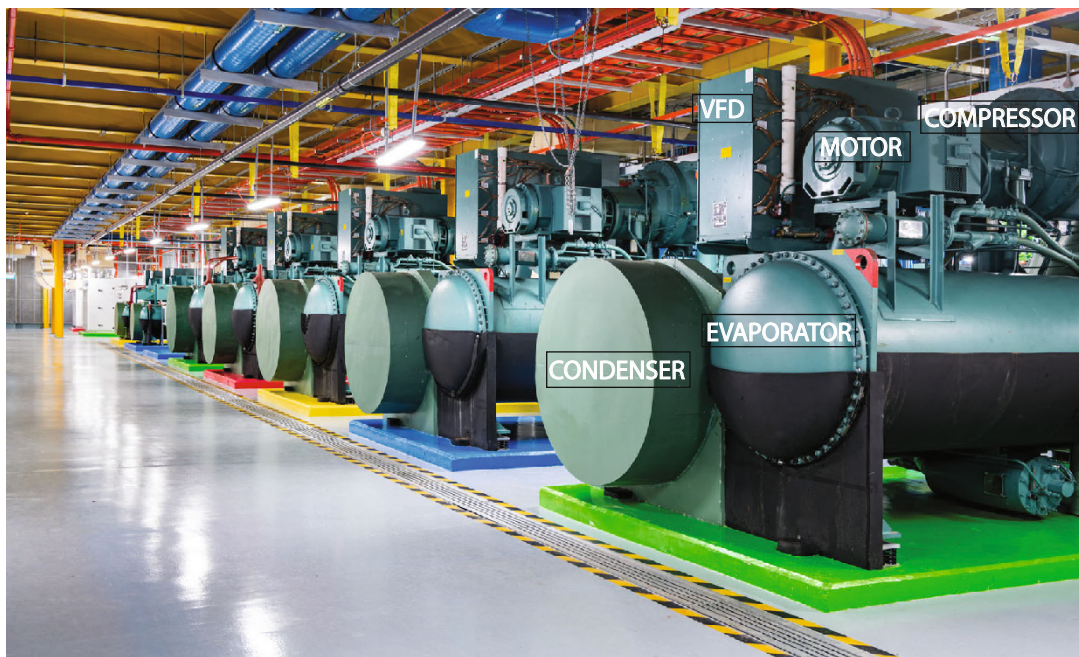
Figure 4.11: Water-cooled centrifugal chiller.
