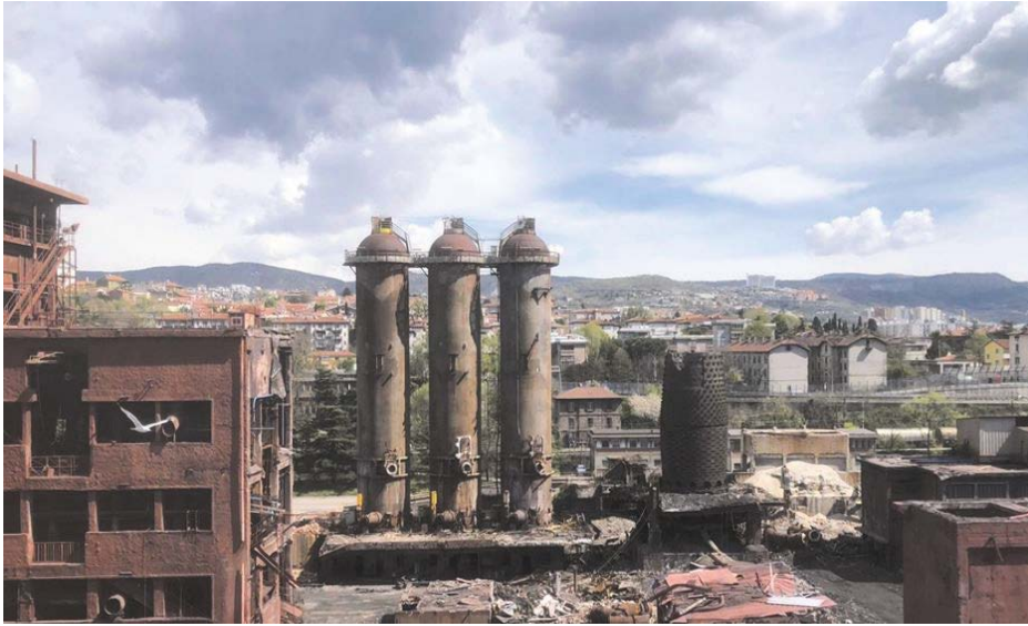
Figure 3 - The hot area of the Servola ironworks undergoing demolition (author's photo, April 2021).
