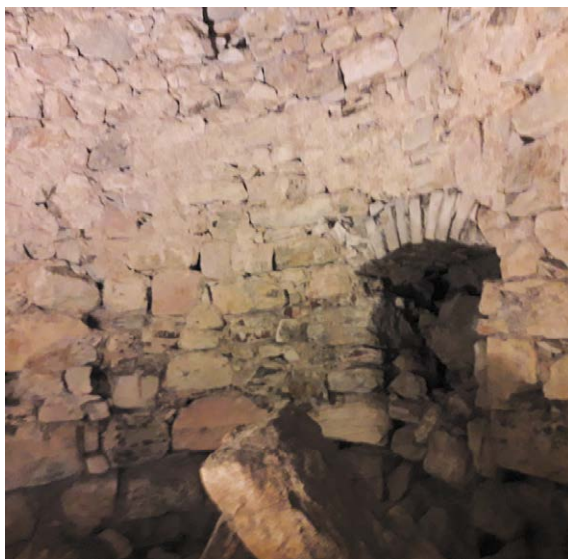
Figure 6 – Underground room at limonaia Fondo Campagnola (Gargnano) to collect and drain the water springing from the rocks.
