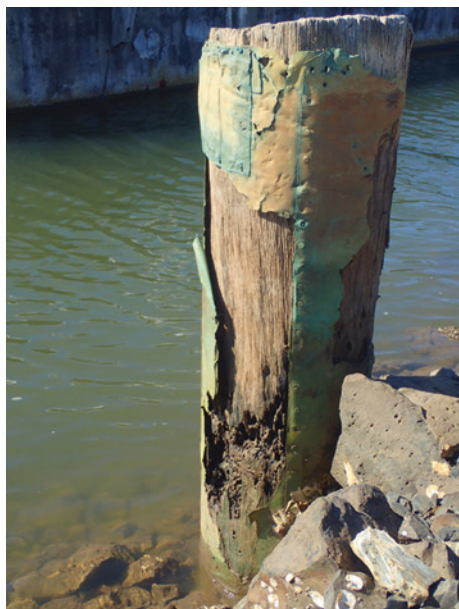
Figure 7.8 Copper sheathing was used to protect pylons prior to the invention of antifouling paints. This metal remains a legacy pollutant (Richmond River, NSW, Australia 2020). Photo: A. Reichelt-Brushett
