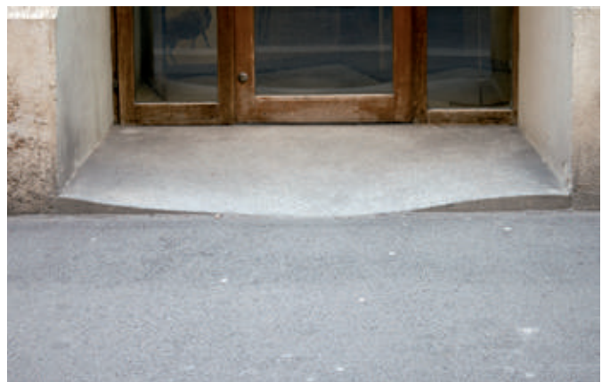
The floor slab near the entrance simulates centuries of wear and tear.
