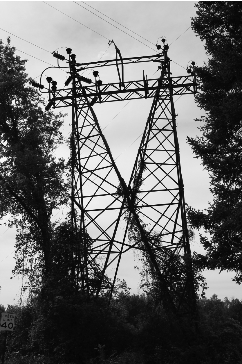
Electric towers in Charlton, New York
