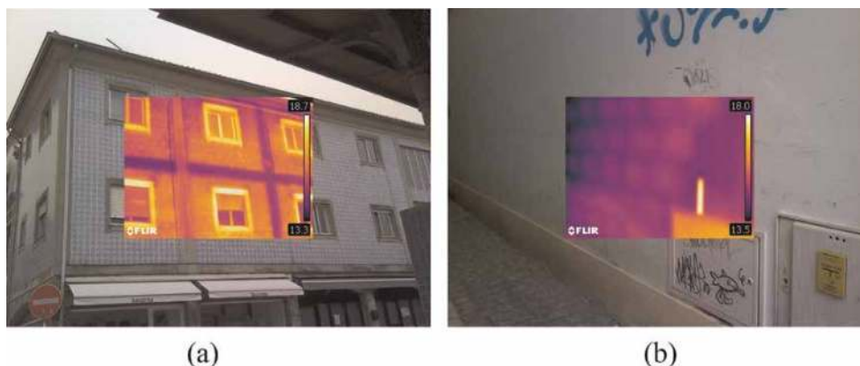
Figure 5. Thermographic survey showing (a) reinforced concrete structure and (b) masonry units with 16 cm ruler as indicated by an asterisk.
