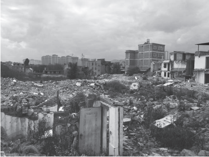
FIGURE 10. A peri-urban village undergoing demolition. Resettlement housing is visible in the background. Photo by author.
