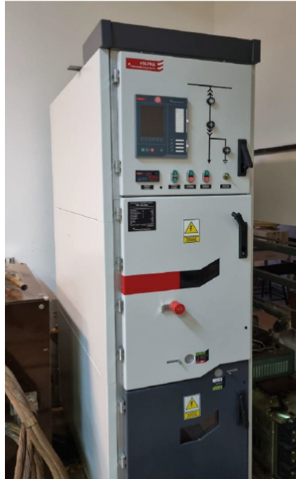
Fig. 1. MV switchgear from Elektrometal Energetyka SA (picture taken in WUT).
