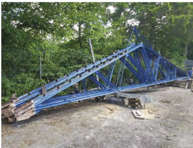
Figure 4. Single storey hall after demolition of inner parts with intact roof. Steel-based roof structure after deconstruction.
