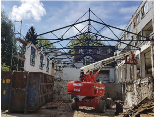
Figure 3. Deconstruction process: All not-bearing parts are removed. The steel-structure will be removed by crane.
