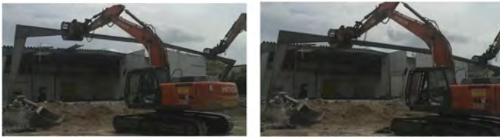
Figure 10. To avoid instabilities, two excavators carefully pull down the structure to the ground.
