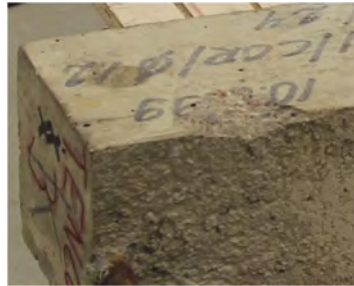
Figure 3. Spalling on the beam.
