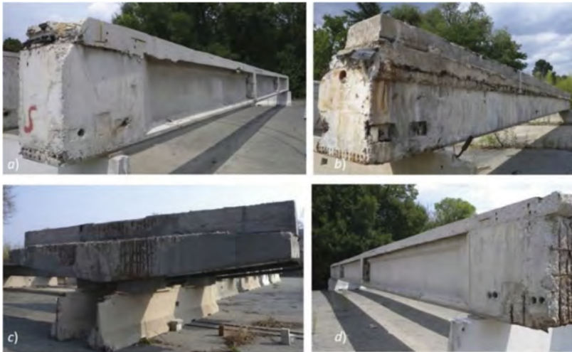
Figure 1. View of different types and condition degradation state of PC structural elements preserved in the testing area. (a) Northern and eastern fronts of I-beam 46-T9-47; (b) Southern and eastern fronts of box-beam 47-C2-SP; (c) Eastern front of pier cap 48; (d) Southern and eastern fronts of I-beam 46-T1-47.
