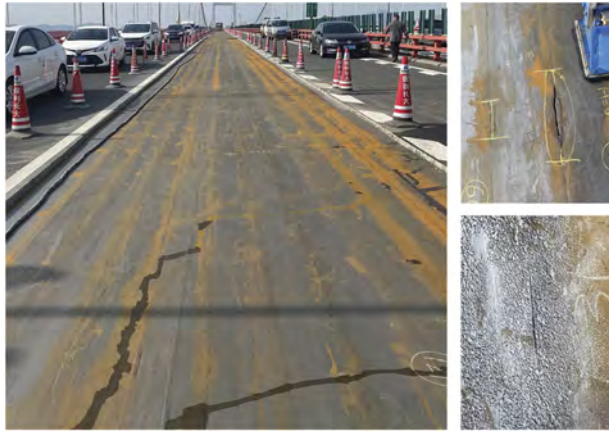
Figure 1. Fatigue cracks on actual OSDs and the corruptions due to pavement damage.
