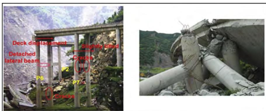
Figure 7. Possible failure mechanism of Baihua Bridge and collapse of the bent 5 (Kawashima, Takahashi, Ge., Wu, Zhang 2009).
