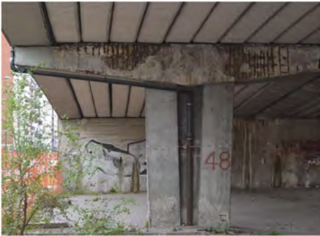
Figure 1. Corrosion-induced degradation of a pier cap of the bridge before dismantling (Biondini et al. 2020).
