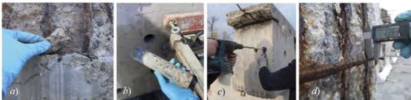
Figure 10. Different sampling procedures during onsite inspections: (a) concrete fragments, (b) concrete cores, (c) concrete powders, and (d) samples of steel reinforcement.
