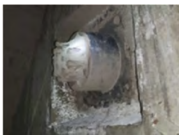
Figure 4. One of the anchorages without proper cap.
