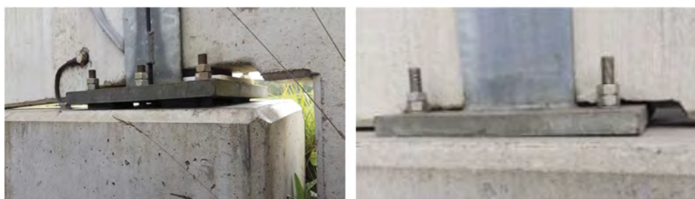
Figure 2. Exemplary photographs of the fastening situation of NB on the concrete edge beam.
