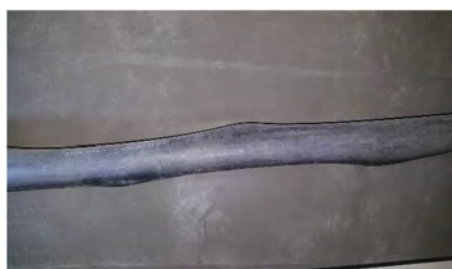
Figure 5. Critical condition of a tendon.
