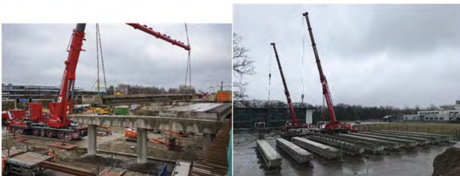
Figure 1. Deconstruction of prefab girders in Groningen (left) and girders in temporary storage (right).
