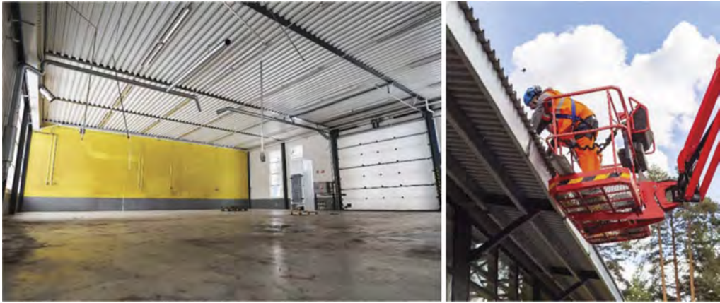
Figure 3. Steel hall in Lämminpää district, Tampere, Finland (left) and its deconstruction (right).
