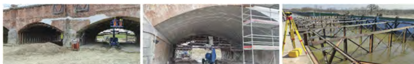
Figure 7. Bridge strengthening: arches renew by cast in situ of lightweight concrete, FRCM intrados of arches, load test on the strengthened spans of the channel with water intake.
