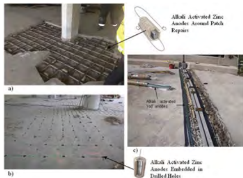
Figure 1. Alkali activated galvanic anodes, (a) as in inset, attached to steel reinforcement prior to the application of the repair material, (b) as in inset, inserted in a grid formation in drilled holes and (c) as 'rods' positioned along steel reinforcement in an expansion joint prior to the placing of the repair mortar.
