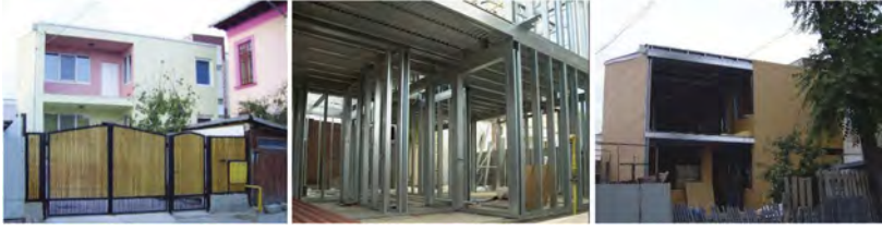
Figure 7. (a) 3D view of the house; (b) steel skeleton; (c) skeleton with structural OSB sheathing.
