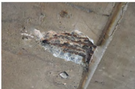
Figure 4. Delaminated concrete removed.
