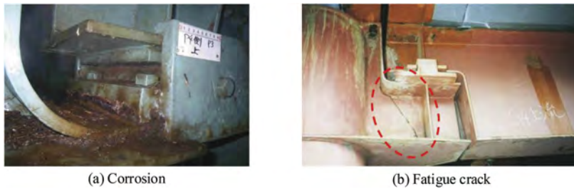
Figure 1. Examples of damage in hinge bearings.
