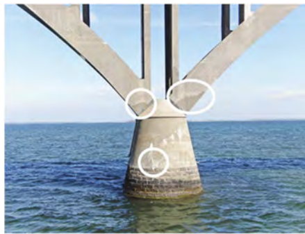
Figure 9. RGB photo of potential delaminated areas on concrete bridge pier.
