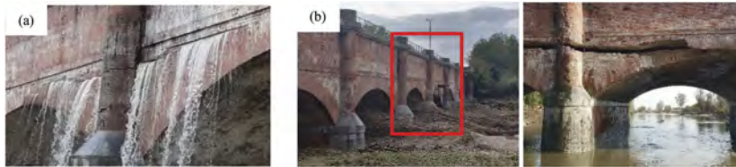
Figure 4. Horizontal crack in the “head wall” downstream (a), and wide horizontal crack in the “head wall” and missing portion of the masonry at the kidneys of the “external” arch and the “head wall” upstream (b).
