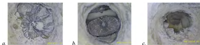
Figure 6. The endoscopy in a. shows a fully grouted duct, the one in b. a void between the duct and the concrete matrix, the one in c. an ungrouted duct.
