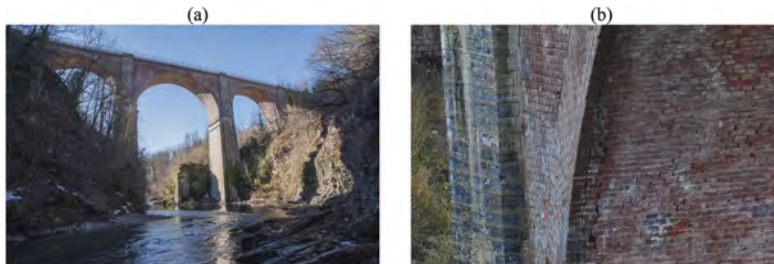
Figure 1. The Olla bridge: (a) picture from the Stura River; (b) existing damages on the second arch.
