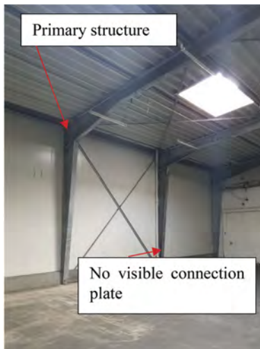
Figure 4. Steel structure: The primary structure is made of 4 arcs of steel. There is no visible connection plate on the ground. Obviously, the columns are poured into the concrete. (left).
