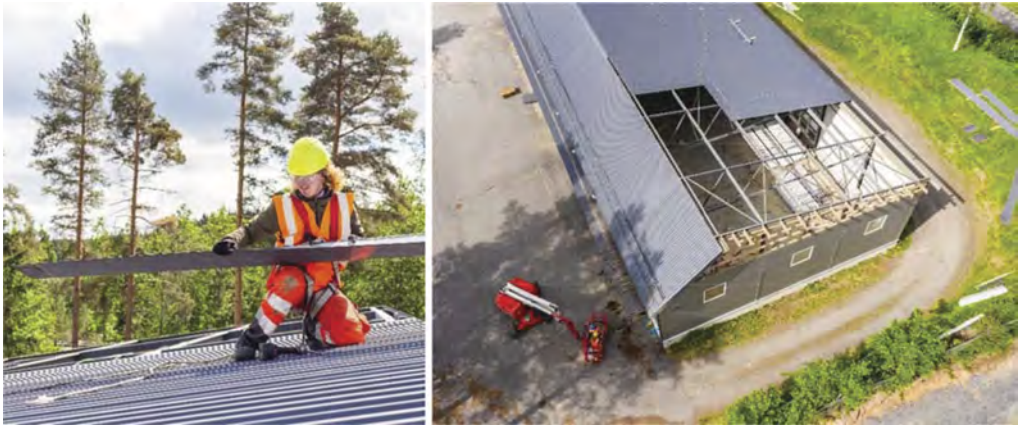
Figure 4. Manual deconstruction of the roof cladding (left) and the aerial view of the deconstruction site (right).
