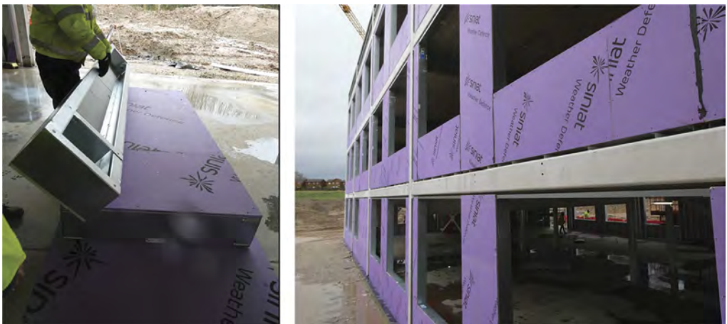
Figure 3. Prefabricated panelised infill wall with exterior plasterboard (photos taken by the authors on December 2021 in the Greater Manchester area, UK).
