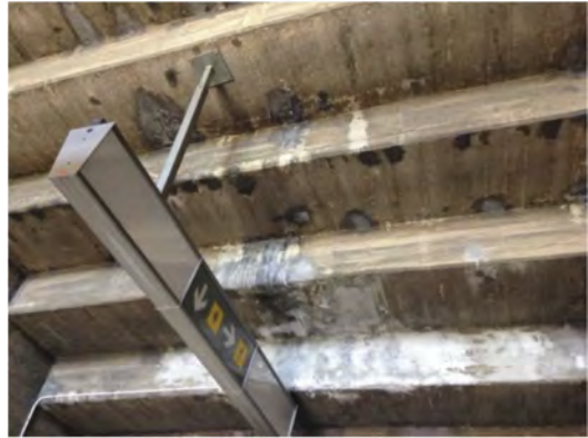
Figure 9. Leaking places underneath the bleachers.
