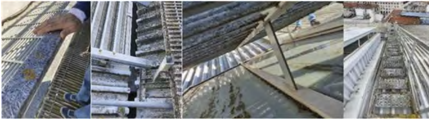
Figure 3. Roof handrails (a); brise-soleil and polycarbonates (b, c); paths and stairs (d).
