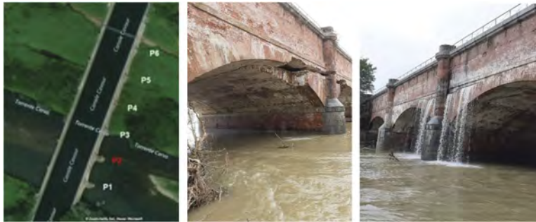
Figure 1. Pile numbering highlighting the P2 pile in which the failure was detected, upstream and downstream damages.
