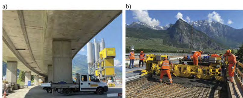
Figure 8. a) UHPFRC ready mix plant next to the Riddes Viaduct, b) UHPFRC casting on the deck slab.
