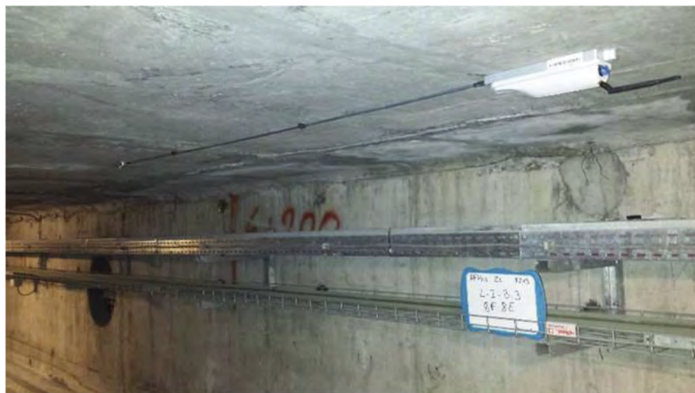
Figure 2. One wireless Optical Strand set under the concrete slab of the Mont-Blanc tunnel.
