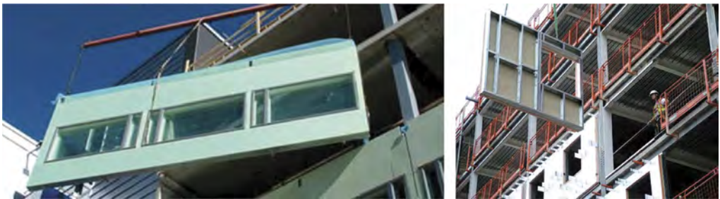
Figure 2. Installation of lightweight infill wall in a primary structural frame (images from SCI, 2008), (left): Prefabricated infill wall with cladding, windows, and light steel frame, and (right) prefabricated infill wall with exterior plasterboard, windows, and light steel frame.
