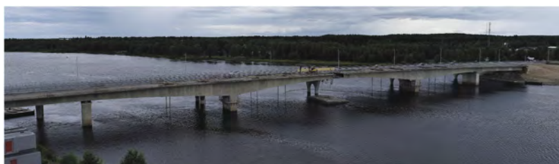
Figure 9. Kalix bridge during demolition, with anchors in place (courtesy of NCC Infrastructure).
