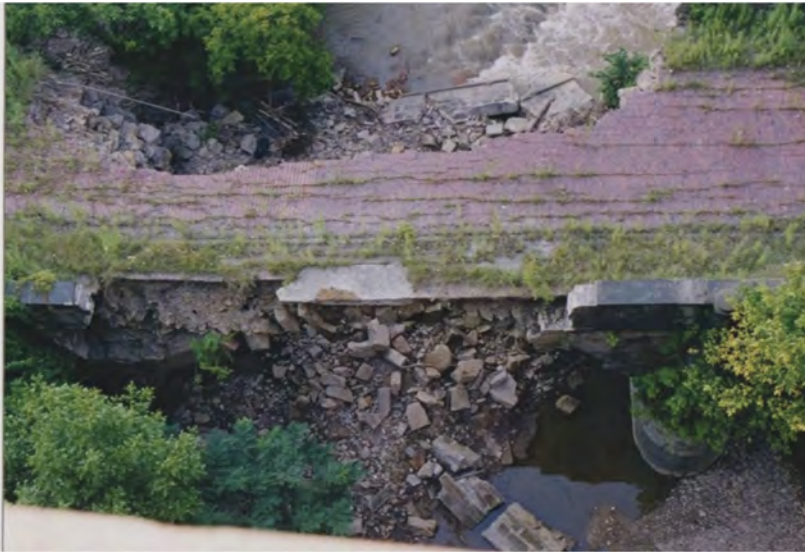
Figure 1. Collapse of Blaine, OH viaduct 1999 (viewed from above).
