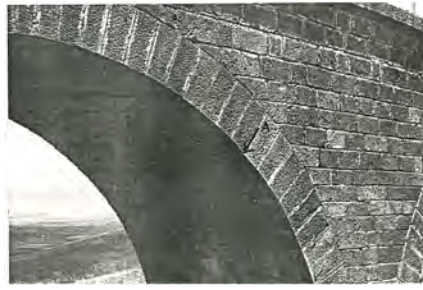
Figure 2. Crack pattern at the haunches of the arch evidenced during the inspection of 1984.
