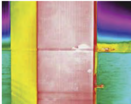
Figure 7. Potential areas with delaminated concrete - captured using thermography.
