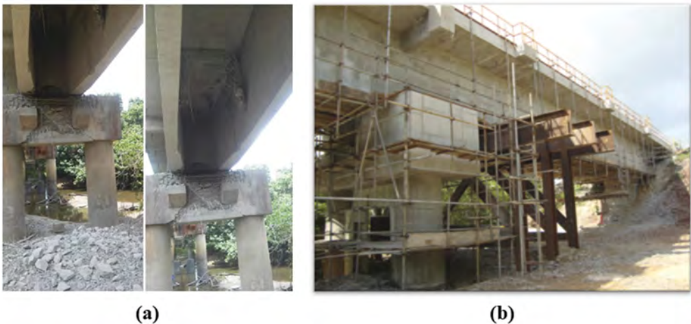
Figure 2. Bridge rehabilitation process: (a) damage caused by an act of vandalism in 2017, (b) process for bridge rehabilitation and strengthening.
