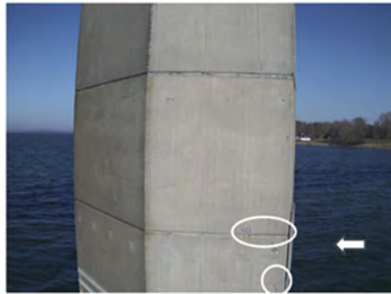
Figure 6. Potential areas with delaminated concrete (verified by rope-access personnel).
