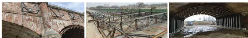
Figure 6. Bridge safety works: belting with steel ropes and internal channel steel truss beams, internal steel ribs similar shape to the wooden type of the original arches construction period.
