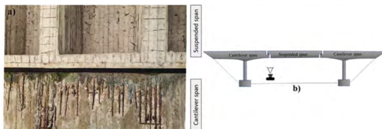
Figure 1. Degradation of an RC bridge's half-joint: a) view from the intrados and b) bridge scheme and viewpoint.
