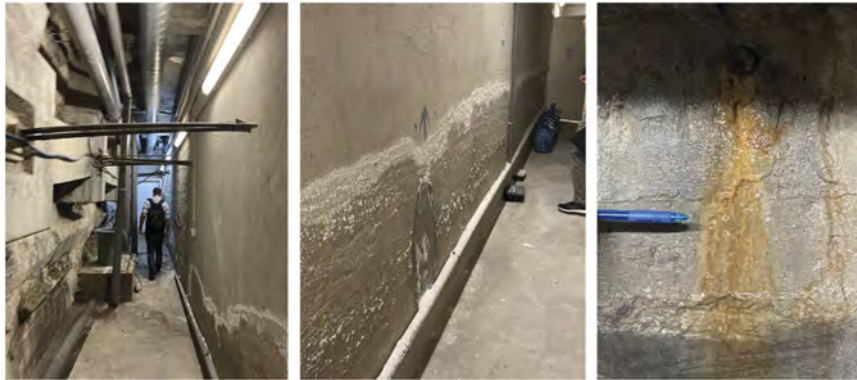
Figure 8. Gallery (a), rising damp and efflorescence (b) and orange-coloured run-off (c).
