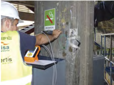
Figure 4. Measuring the corrosion in a column.
