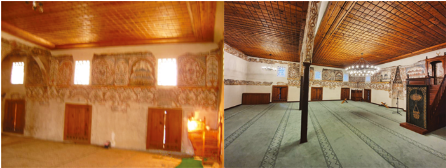
FIGURE 6.23 Inner image of north-east wall in 2005 (left) and after restoration in 2021 (right-KMSH)
