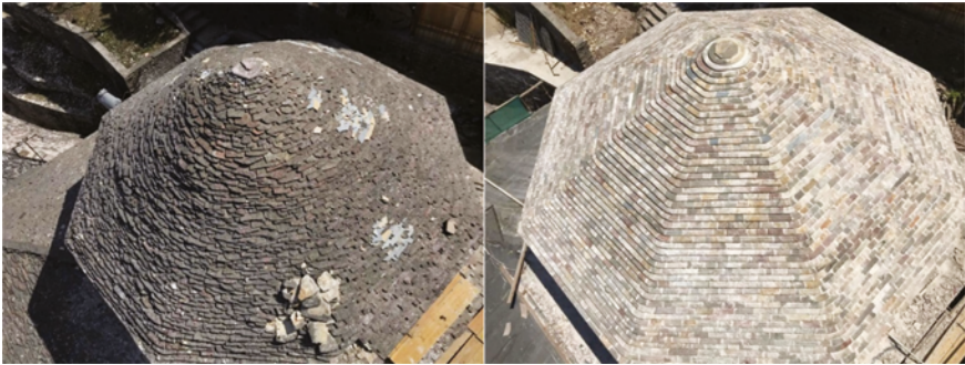
FIGURE 6.28 The dome of the Mosque of Bazar before restoration (left- FMTK) and after restoration (right- FMTK)
