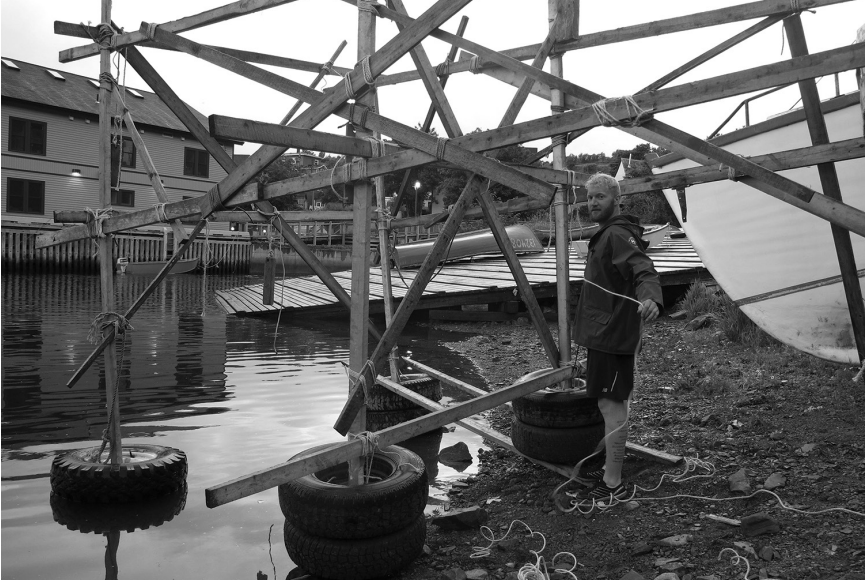
Figure 8.13: Traveller Bradley Peters lashing together the framework of the “Quidi Vidi Camera Obscura,” Art Marathon, St. John’s, Newfoundland, 2014. Source: Author
