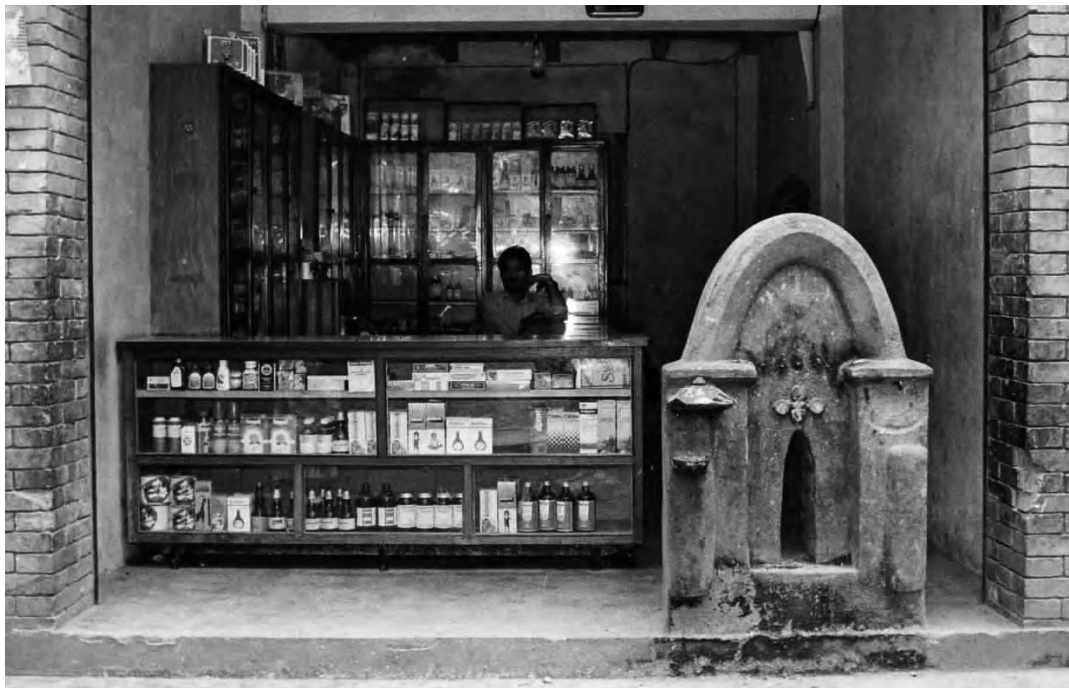
Fig. 7: Haimāpvaḥ in Gvaḥmādhī 1995. After demolition of the old brick house the flight lane of Haimāḍyaḥ had to be preserved in its original position in front of the new medical store and received a cement finial.
