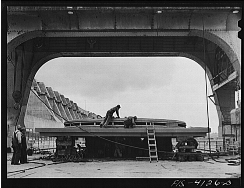
Figure 25.3 “Cherokee Dam, Tennessee, Tennessee Valley Authority. Working on the cover of a 30,000 kilowatt generator under a 250 ton gantry crane,” photographed by Arthur Rothstein, June 1942. Like other photographs sponsored by the Farm Security Administration, this image celebrates the people who built infrastructure.
