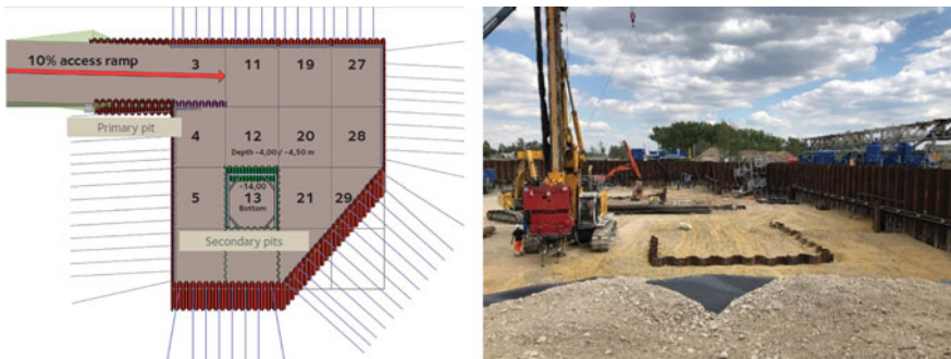
Fig. 3.5 Left: Plan view—Excavation pit; Right: Installation of sheet piles for the secondary excavation pit [18]
