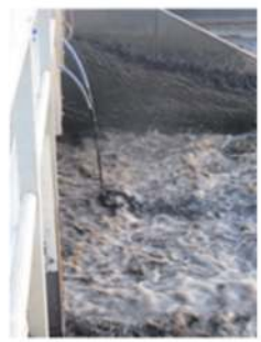
PAC dosing @ oxidation ditch
