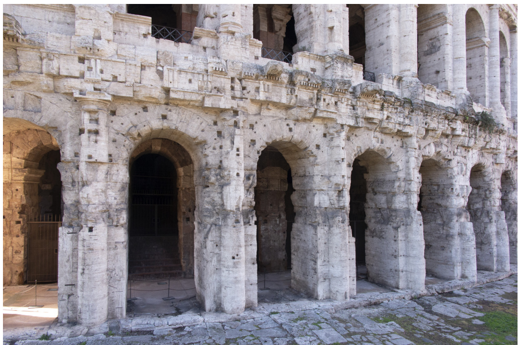
Fig. 5. Detail of the first order of the Theatre of Marcellus showing the different state of conservation of the lower portion of the pillars. Photography by the authors.
