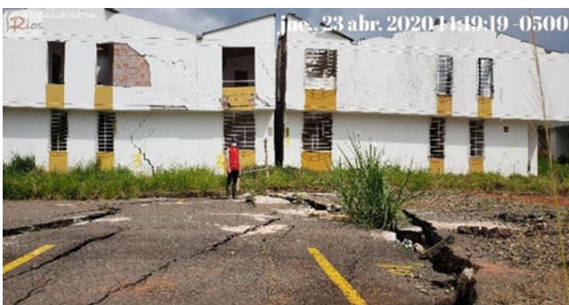
Fig. 13 Crack evolution on July 1st (20 days after the landslide)
