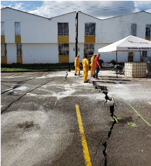
Fig. 12 First cracks appeared on June 12, 2019 (One day after the landslide) in block Mz5, 80 m far from the main scarp, as indicated in Fig. 11
