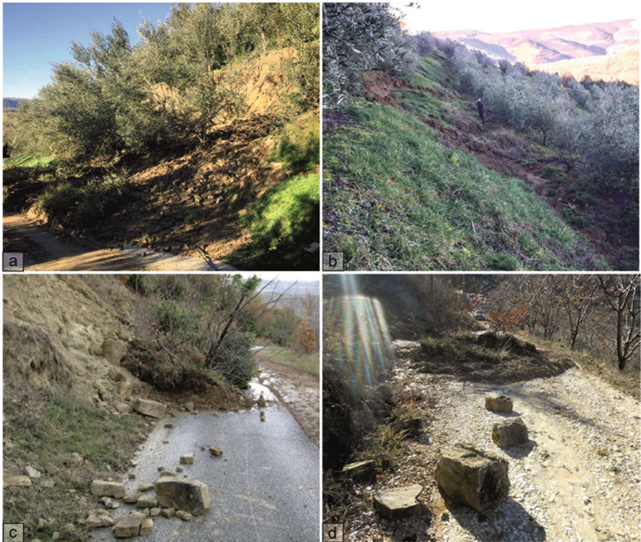
Fig. 3 Landslides activated in December 2020 in the Istrian flysch area
