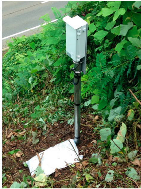
Fig. A.43 Example of sensor installation
