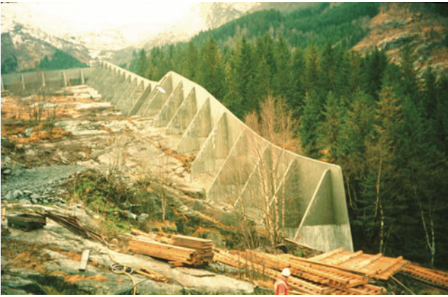
Fig. 3 Example of Reinforced Concrete (RC) wall used as diverting dam against snow avalanches at Odda, Norway (Barbolini et al. 2009)
