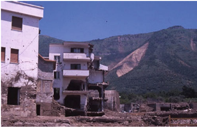
Fig. 1 Example of damage to non-structural elements caused by the impact of flow-like landslides in the Sarno area, Campania, southern Italy, 1998 (from Mavrouli et al. 2014)
