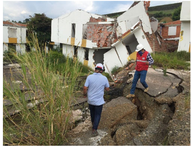
Fig. 14 Total damage observed in block Mz 5 on July 21, the same day of occurrence of the second landslide
