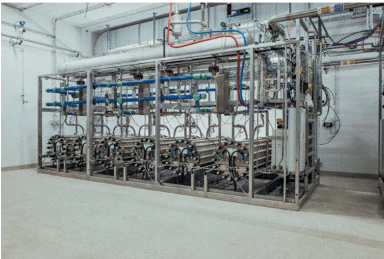
Figure 9.7: One of the electrolyser systems. (Source: Maximilian Kamps, Agentur Blumberg GmbH)
