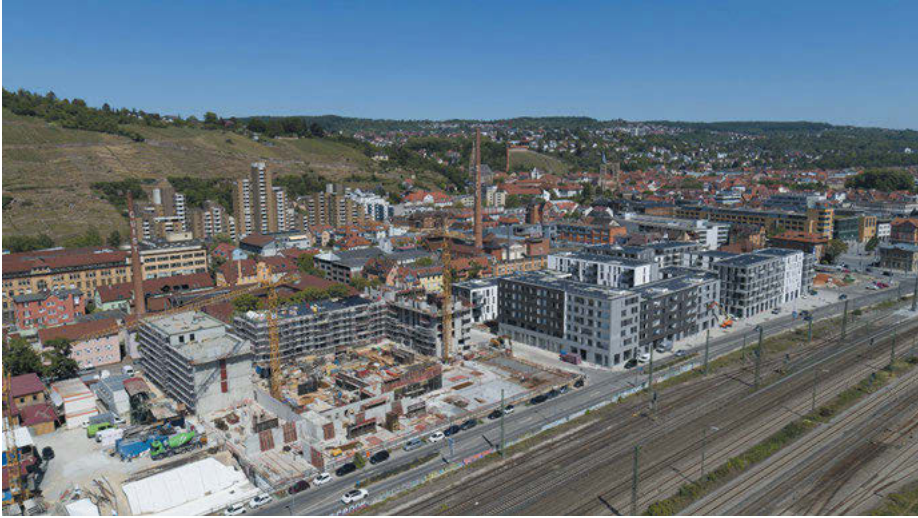
Figure 9.5: “Klimaquartier Neue Weststadt” in May 2020 with the finalized building blocks B (far right) and C (right) and block D (“Desiro”, left) under construction against the backdrop of Esslingen’s vineyards, Weststadt and historic district. (Source: Maximilian Kamps, Agentur Blumberg GmbH)
