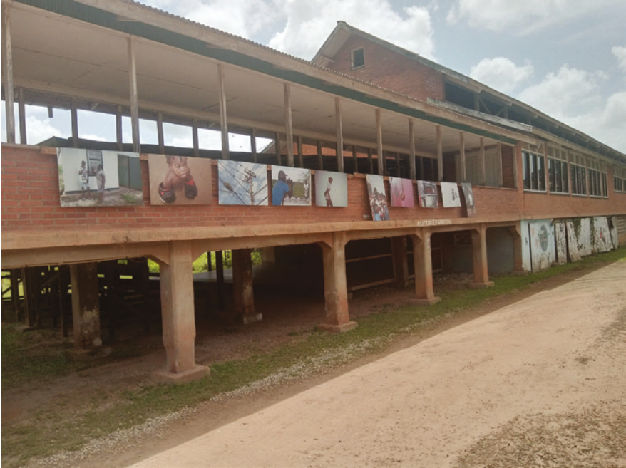
FIGURE 6.1 Moengo's hospital, currently in a state of disrepair and used as an art exhibition space
