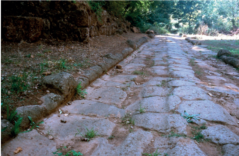
Figure 1.2 Half-paved road width on the Via Amerina south of Falerii Novi, Italy. © Ray Laurence.
