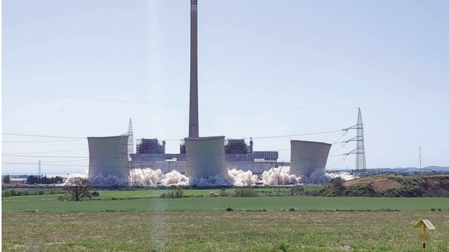
Fig. 2 Cooling towers of the Andorra thermal power plant being demolished on 13 May 2022. Photo courtesy of Andorra City Council
