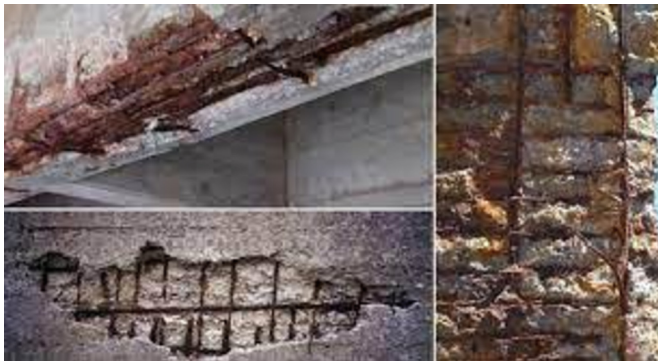
Fig. 3. Corrosion in concrete structures (Murari et al. 2021).
