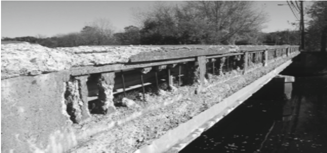
Fig. 1. A concrete bridge parapet wall exhibits severe deterioration caused by repeated freezing and thawing cycles (Susca 2006)
