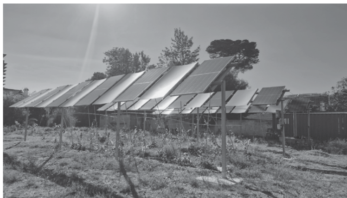
Figure 8.1: Agrivoltaics facility installed at the University of Lisbon
