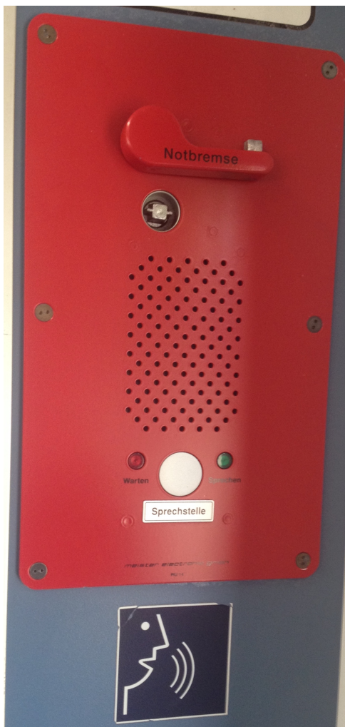
Figure 3-15. Intercom system in German regional trains using a half-duplex transmission mode. The user is required to wait with the red light and may talk when the green light flashes (Source: Christoph Oemig).
