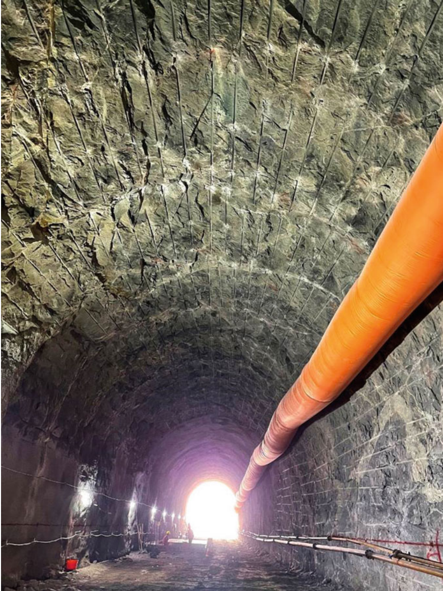
Fig. 2.12 Very good quality of the rock mass after drill-and-blast excavation of the ramp
