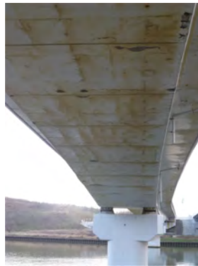
Fig. 5. Bridge redeterioration due to chloride attack after repair near Noto Peninsula (Note that the picture was taken in 2017 by the second author)
