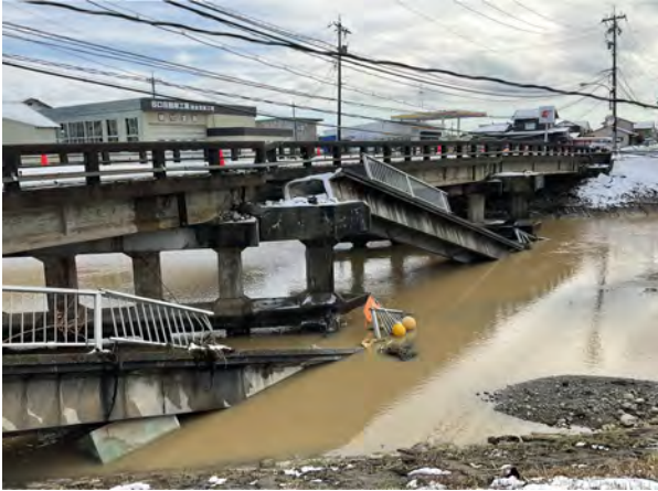
Fig. 2. Sidewalk collapse of Ukai Bridge subjected to ground motion and/or tsunami caused by 2024 Noto-Hanto earthquake. Note that the picture was taken by the second author.
