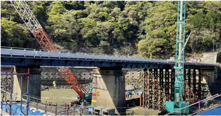
Fig. 9. Washout of superstructure due to the 2020 Kyushu flood and reconstruction of temporary bridge using the survived bridge piers in Kuma River. Note that the picture was taken by the second author.
