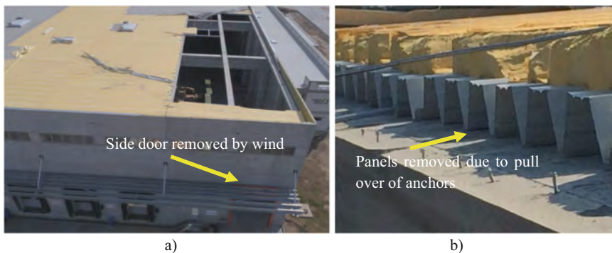
Fig. 15. Roof (and side door) destroyed by wind: a) aerial view with the damaged roof; b) detail with end support fasteners in the affected roof area.
