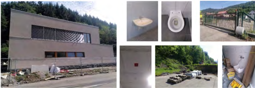
Fig. 1. Picture of the finished the administrative building of Schirmeck (left), pictures of the re-used material (right).
