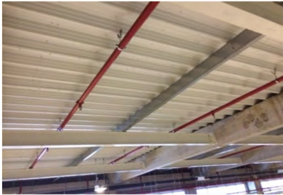
Fig. 17. Retrofitting intervention for roof, with new intermediate secondary IPE steel beams fixed between two concrete purlins and Z steel purlins (top) and photo after completion (bottom).
