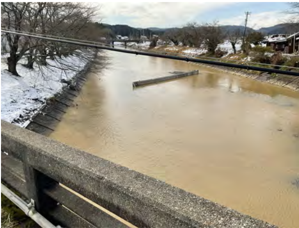
Fig. 3. Washout of Ukai Bridge sidewalk due to tsunami caused by the 2024 Noto-Hanto earthquake. Note that the picture was taken by the second author.
