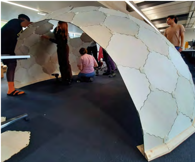
Fig. 2. The ECHO shell during construction. The panels require some external support during assembly, to counteract bending moments; however, support can be removed after assembly.
