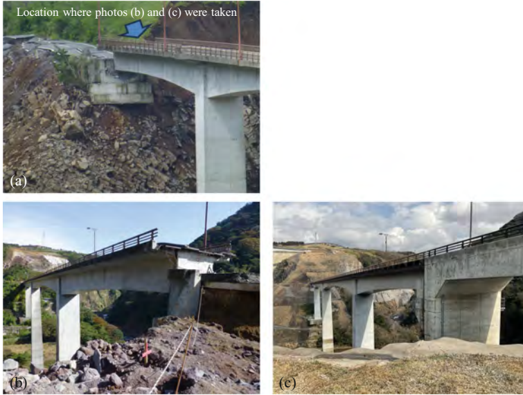
Fig. 8. Example of robust structures against catastrophic hazards (a) and (b) taken after the 2016 Kumamoto earthquake; and (c) taken after the reconstruction of the abutment. Note that all pictures were taken by the second author.
