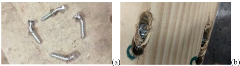
Fig. 5. a) Screws developing a plastic hinge, b) extent of damage in timber.
